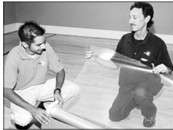
WINDOW PROTECTION: Abid Quraishi, left, and Doug Corrier roll out and measure Hurricane Film Ultra High Performance Safety and Security Window Film to be applied on windows.
